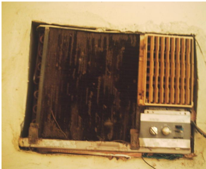
Fig. 1. Evaporator coil before cleaning
