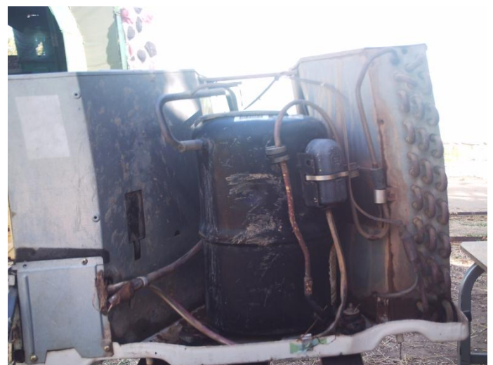
Fig.4. Compressor and condenser coil after cleaning
