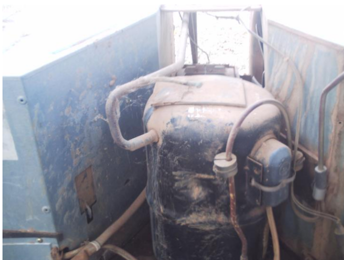
Fig.3. Compressor and condenser coil before cleaning
