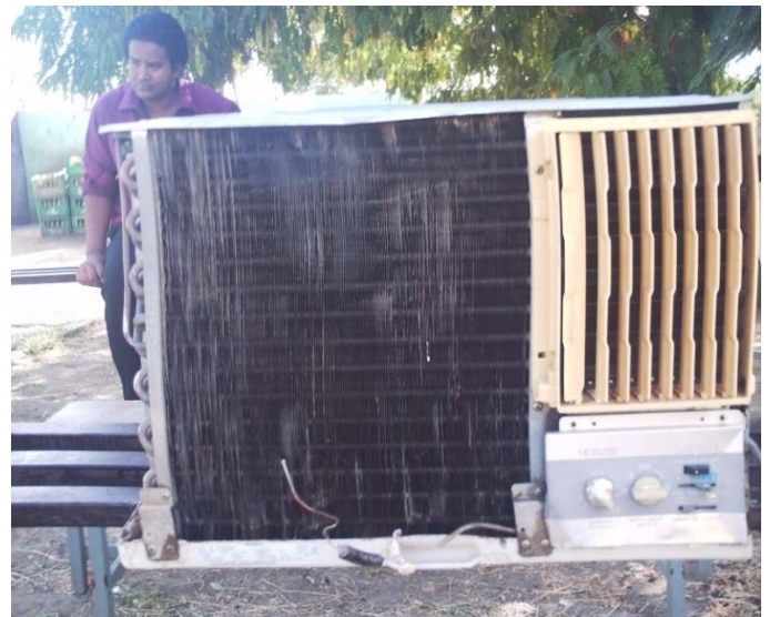
Fig.2. Evaporator coil after cleaning
