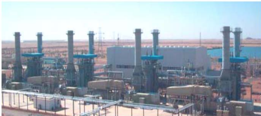
Fig. 4-1 Garri Power plant, 330 MW
