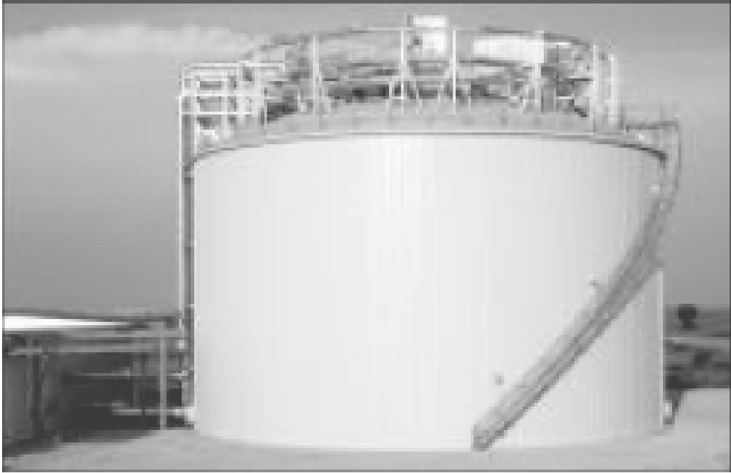
Fig. 4-12 Mueller Avalanche Ice Thermal Storage Tank with Ice harvester on the top of Tank, Lincoln, Nebraska U.S.A [25].
