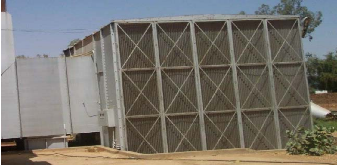
Fig. 2-9 Kilo X South of Khartoum, gas turbine plant box type filter location
