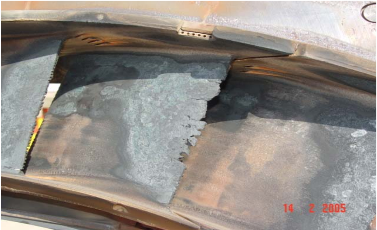
Fig. 2-7 The effects of plugging first stage nozzle cooling passage.
