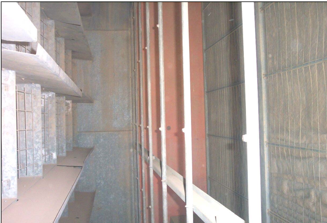
Fig. 4-8 Location of fogging nozzle in filter house
